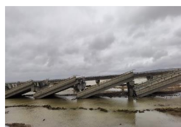
(c)青海玛多地震桥梁坍塌
